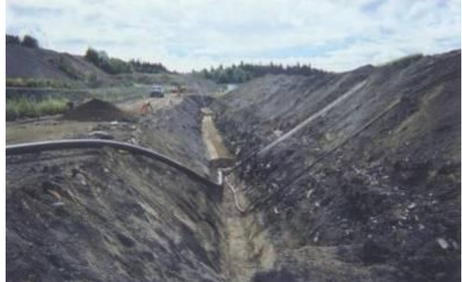
Foothills Boulevard Landfill – installation of gas extraction piping. Source: Wayne Watson Construction Ltd.
